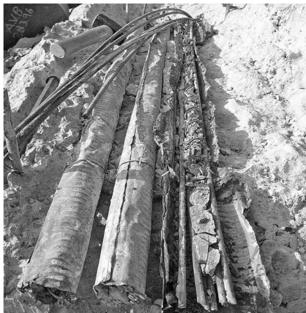
Geöffnetes, schlecht injiziertes Spannglied. Opened tendon with insufficient grouting.
