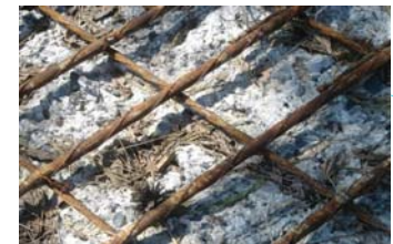
Corroded Reinforcement Bars
