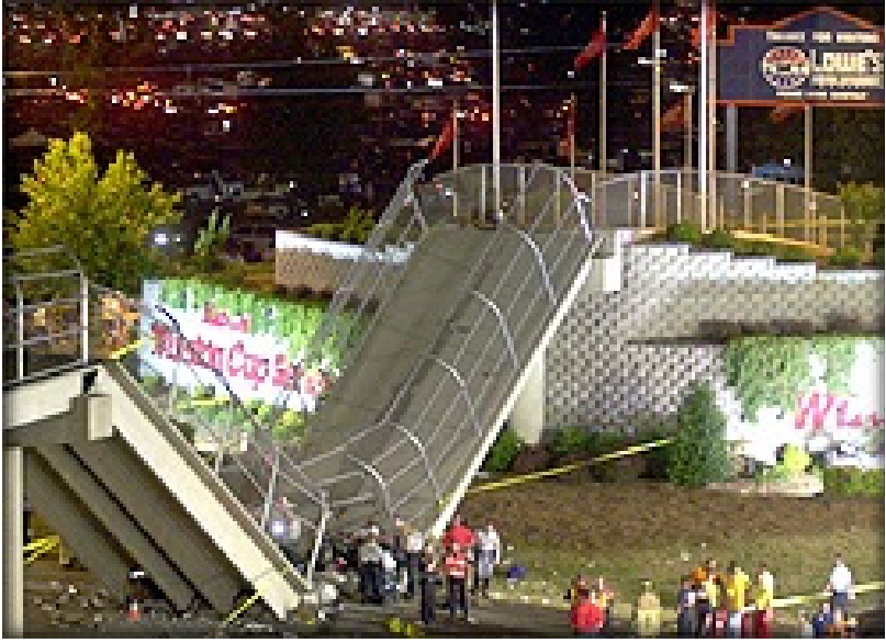
Figure 4.11: Example of collapse of a pedestrians bridge due to pitting corrosion of tendons, Concorde, USA 2000.
